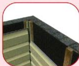
fig 9.1 Showing female component of 2-part corner trim being applied once cladding is finished
