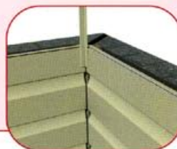
fig 9.2 Showing the male component of 2-part corner trim being applied once cladding is finished
